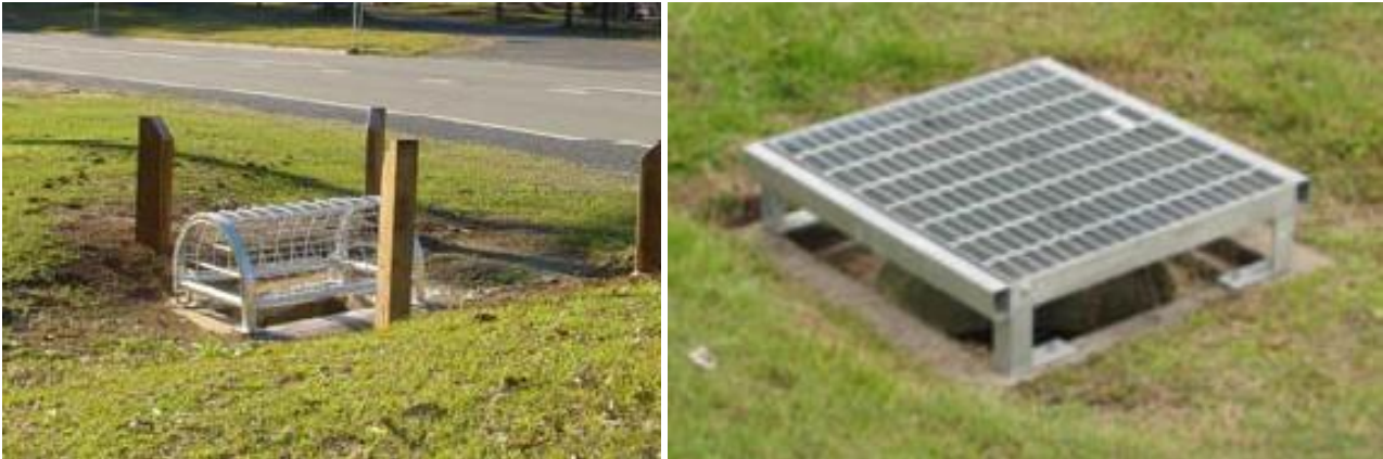
Figure 4.120: Raised drainage cover and wooden bollards
