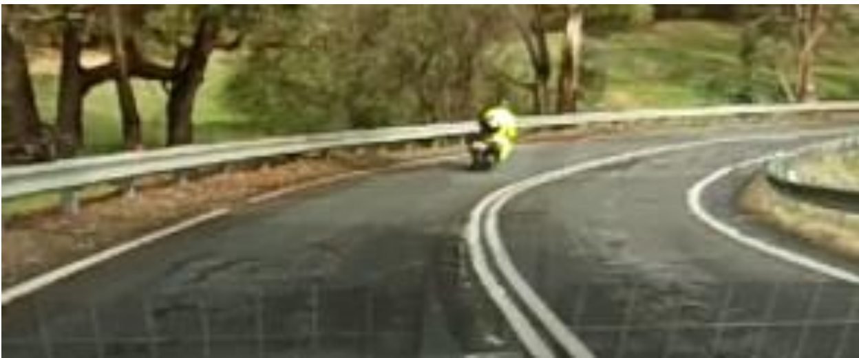
Figure 4.65: Deteriorated pavement on curve (ravelling and stripping)
