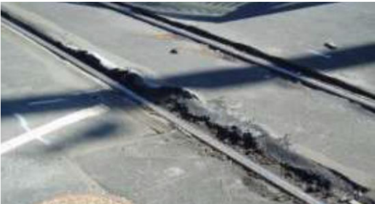
Figure 4.73: Railway crossing, road surface hazards
