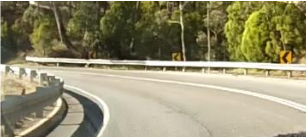
Figure 4.114: Unprotected guardrail posts on outside of curve
