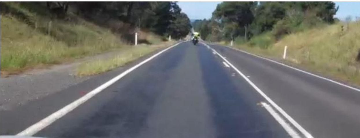
Figure 4.48: Bitumen flushing in the wheel paths
