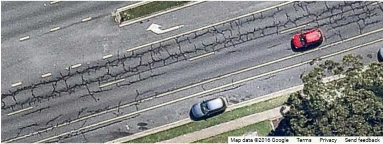
Figure 4.50: Excessive amount of crack sealant
