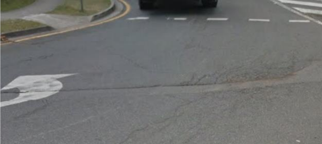
Figure 4.67: Sunken pavement (after trenching) across left turn lane
