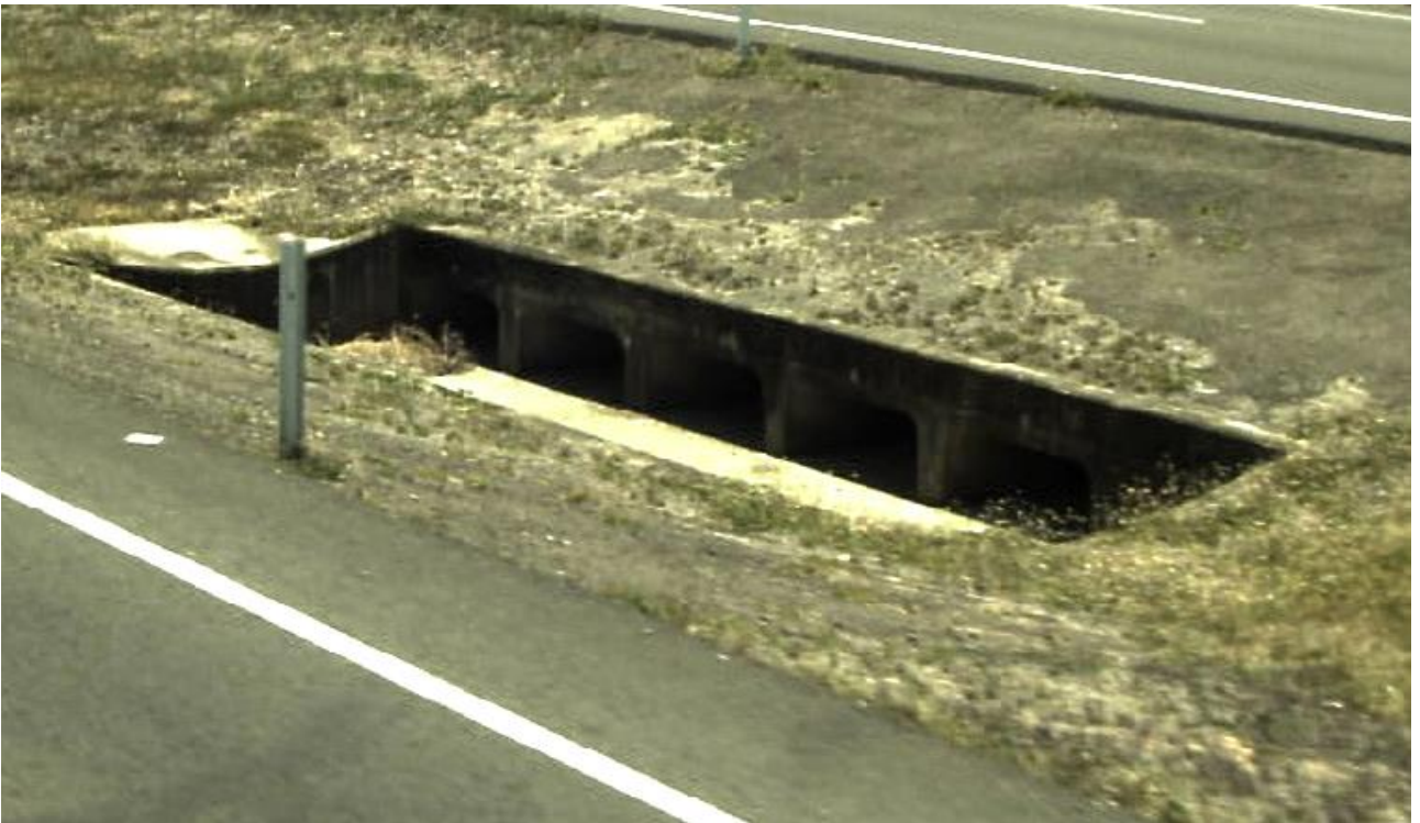
Figure 4.119: Culvert drop in centre median
