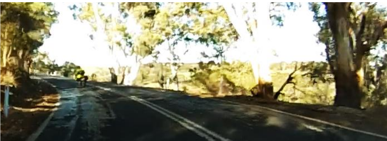
Figure 4.49: Aggregate stripping on curve
