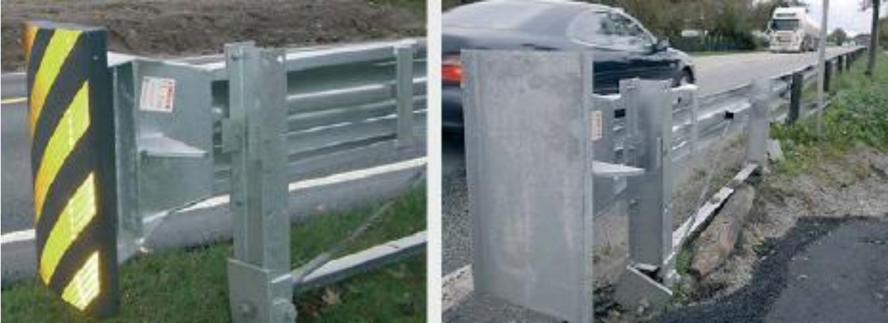
Figure 5.16: Guardrail – ET2000 with and without cover over sharp edges
