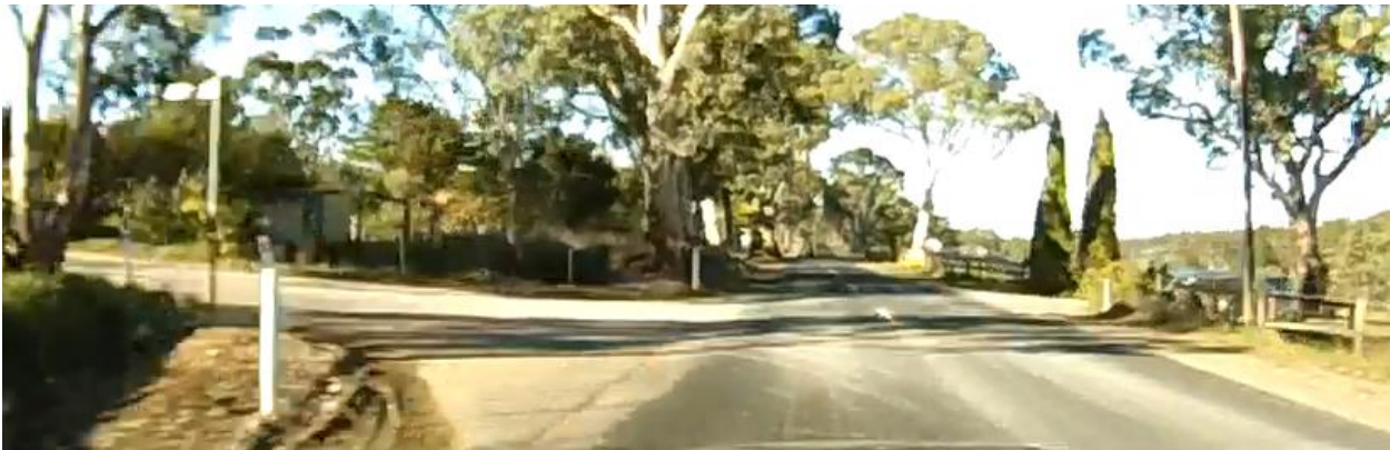
Figure 4.54: Debris on road from unsealed side road
