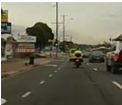
Longitudinal crack on intersection approach
