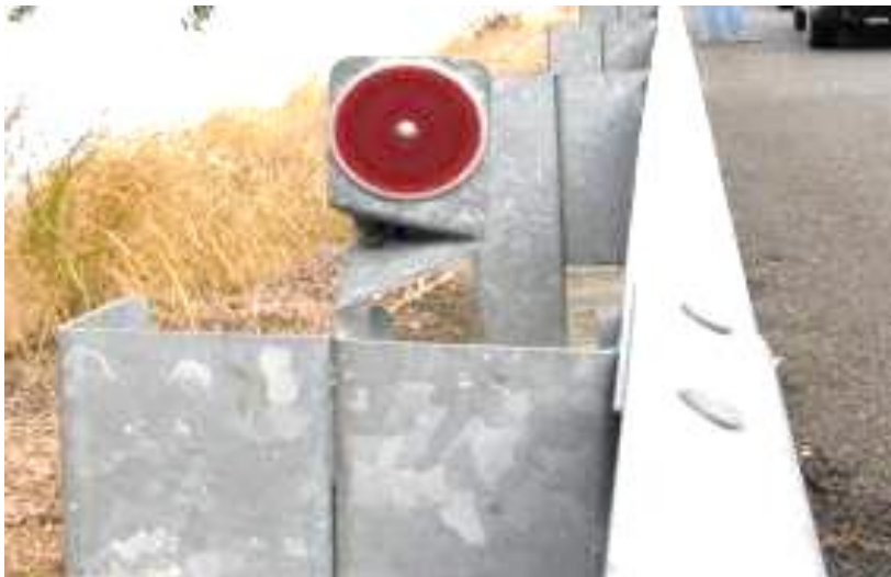
Figure 4.110: Sharp edges on guardrail post tops and metal delineators
